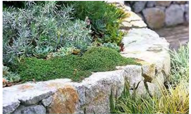
Retaining visible from the street are to be landscaped. *image provided by Seed Landscapes.
