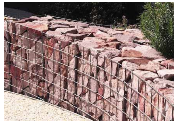
Figure B35 - Gabions with red scoria rock as required on access streets*
