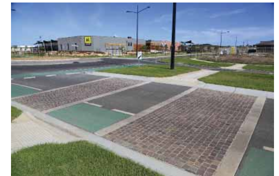
Figure B30 - Porphyry stone thresholds at roundabouts*
